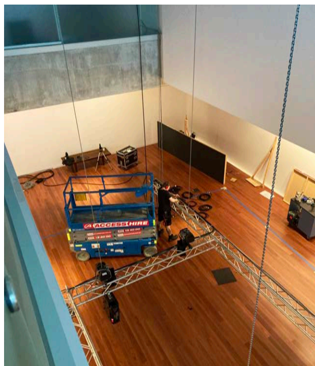
Figure 14. View from above during install - showing the audio visual rigging being prepared prior to hoisting up above the gallery space, Image: Jaquie Hagan
