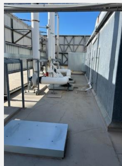
Lower level plant
