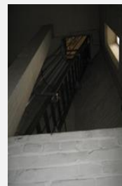
Fixed caged ladder
