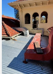
Plant outside roof hatch
