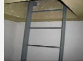
Fixed Ladder access level 6
