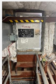
Roof access door
