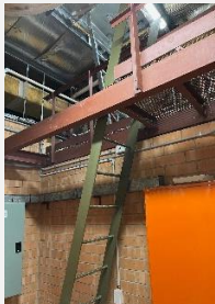
Plant room platform
