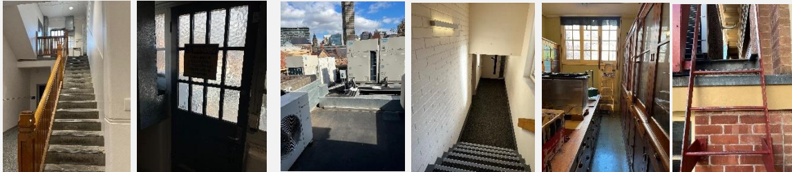
Stairs Access to plant level 1 Plant (level 1) Store room door Access to platform Plant ladder (Grant Kerr)
