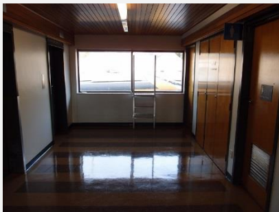
Hughes level 8 access
