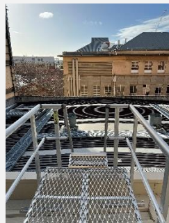
Platform and walkway
