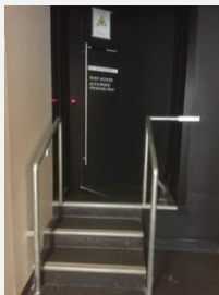
Roof access door
