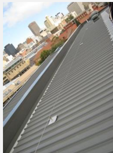
Fall arrest; Western roofs
