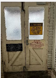
Roof access door
