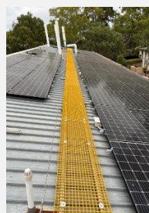
Walkway and static line
