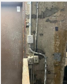
Light switches (East)
