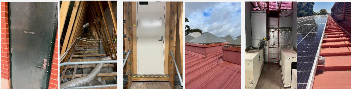
Plant room door Walkway Door to roof access Skylights Ladder to roof hatch Static line
