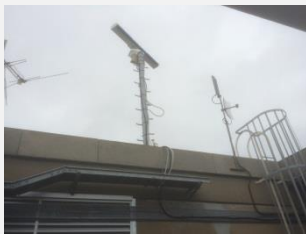
Aerial / antennas etc
